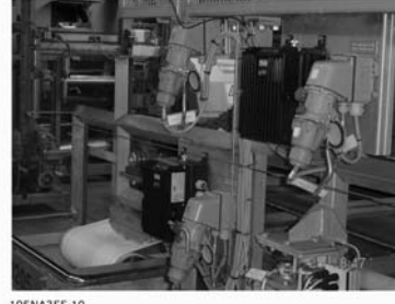
Figure 1.17: Efficient space utilization in the food industry with decentralized motor controls from Danfoss
